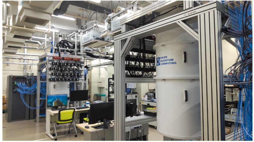
144-qubit superconducting quantum computer “A-II” (front right) and a testbed system (back left)
